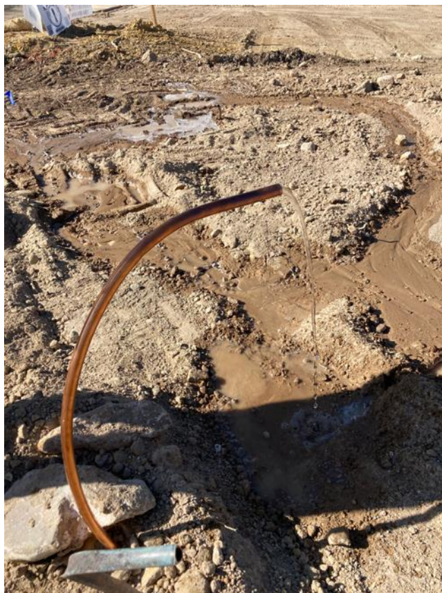
Figure 6. Sampling an accessible service line at a destroyed structure
