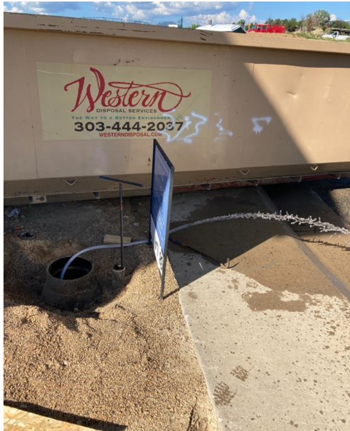
Figure 7. A meter pit being flushed after stagnant sample collection
